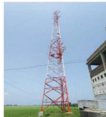
Figure 4: EWDS (Alert Siren) at Donuku, Andhra Pradesh
