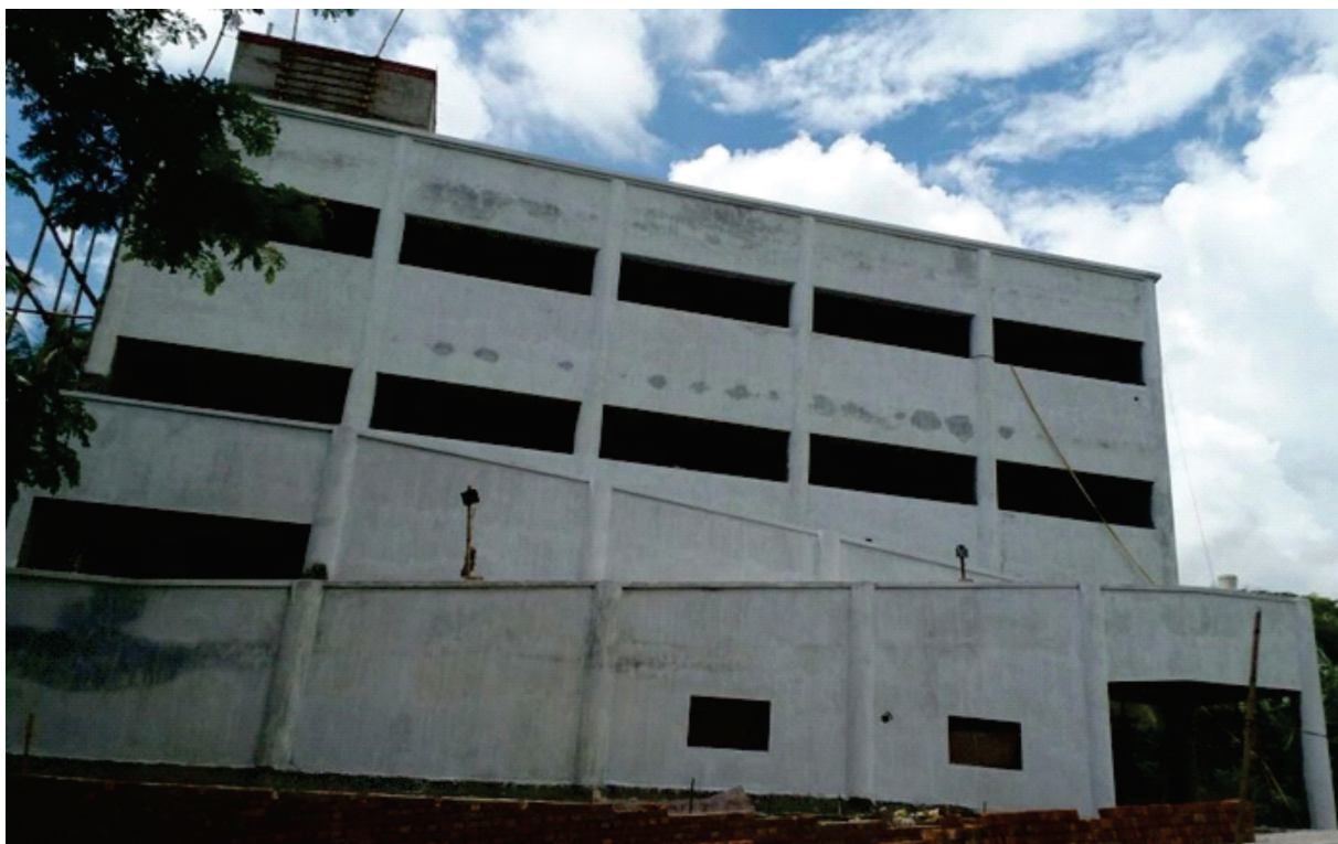
Construction of Cyclone Shelter under at Balisai Kanya Vidyalaya in East Medinipur District.
