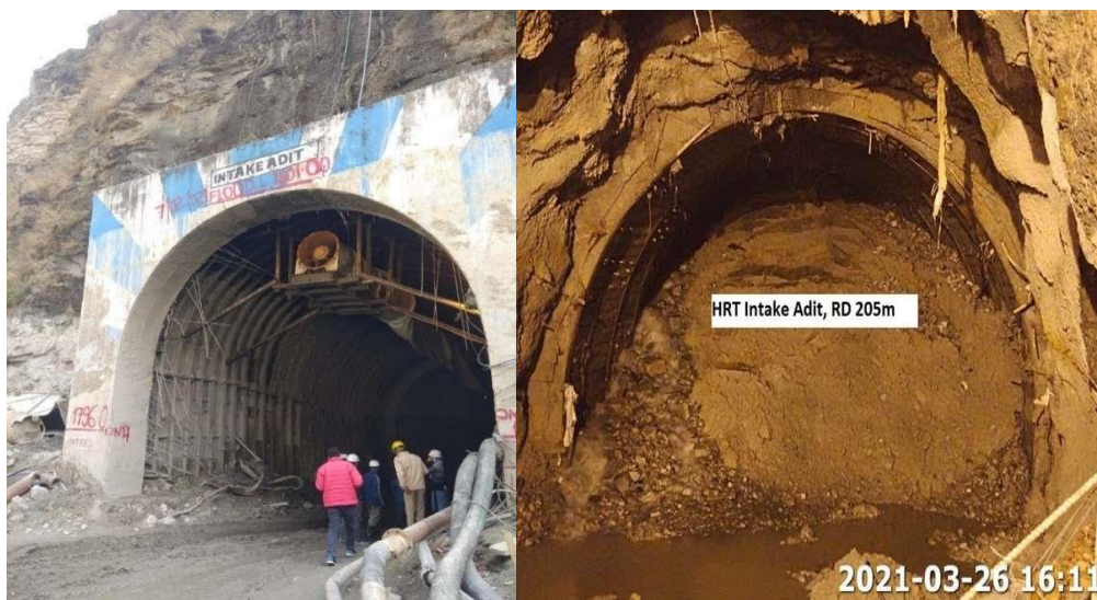
Photo Plate 6: Outside of the intake Adit tunnel with HFL of 1801 m with submerged inside of the HRT intake adit
