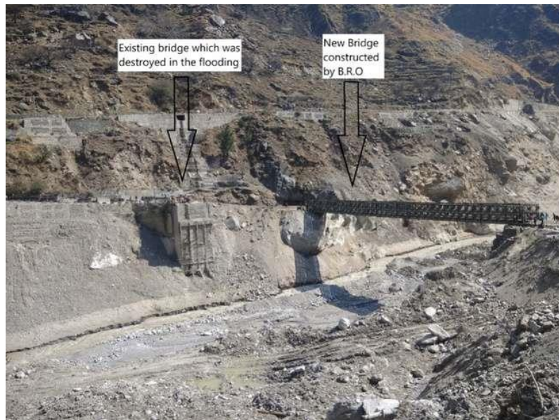
Photo Plate 2: Remnants of damage BRO motor bridge with bailley bridge constructed by BRO for vehicular movement on Joshimath – Malari road after the event
