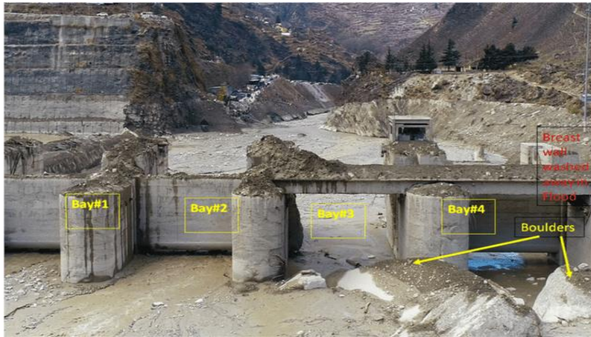
Photo Plate 5: Damaged barrage of NTPC Tapovan-Vishnugad HEP
